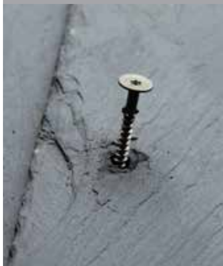
*CUPACLAD™ invisible system uses size 40x20, CUPA PIZARRAS natural slates laid horizontally.
